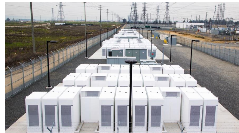
Hornsedale Battery, 220 km N of Adelaide
